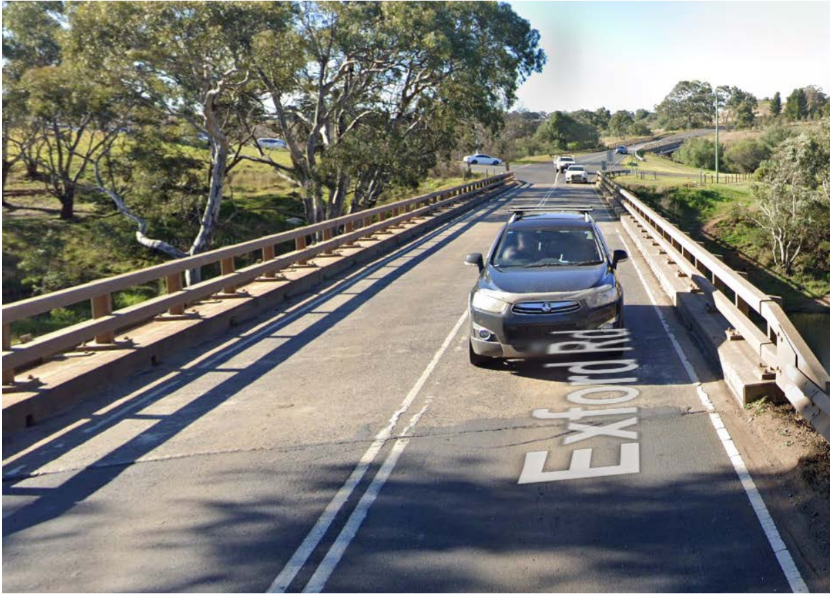
Figure 2 – Exford Road Bridge Site with Greigs Road bridge in the background. Google Street View July 2021
