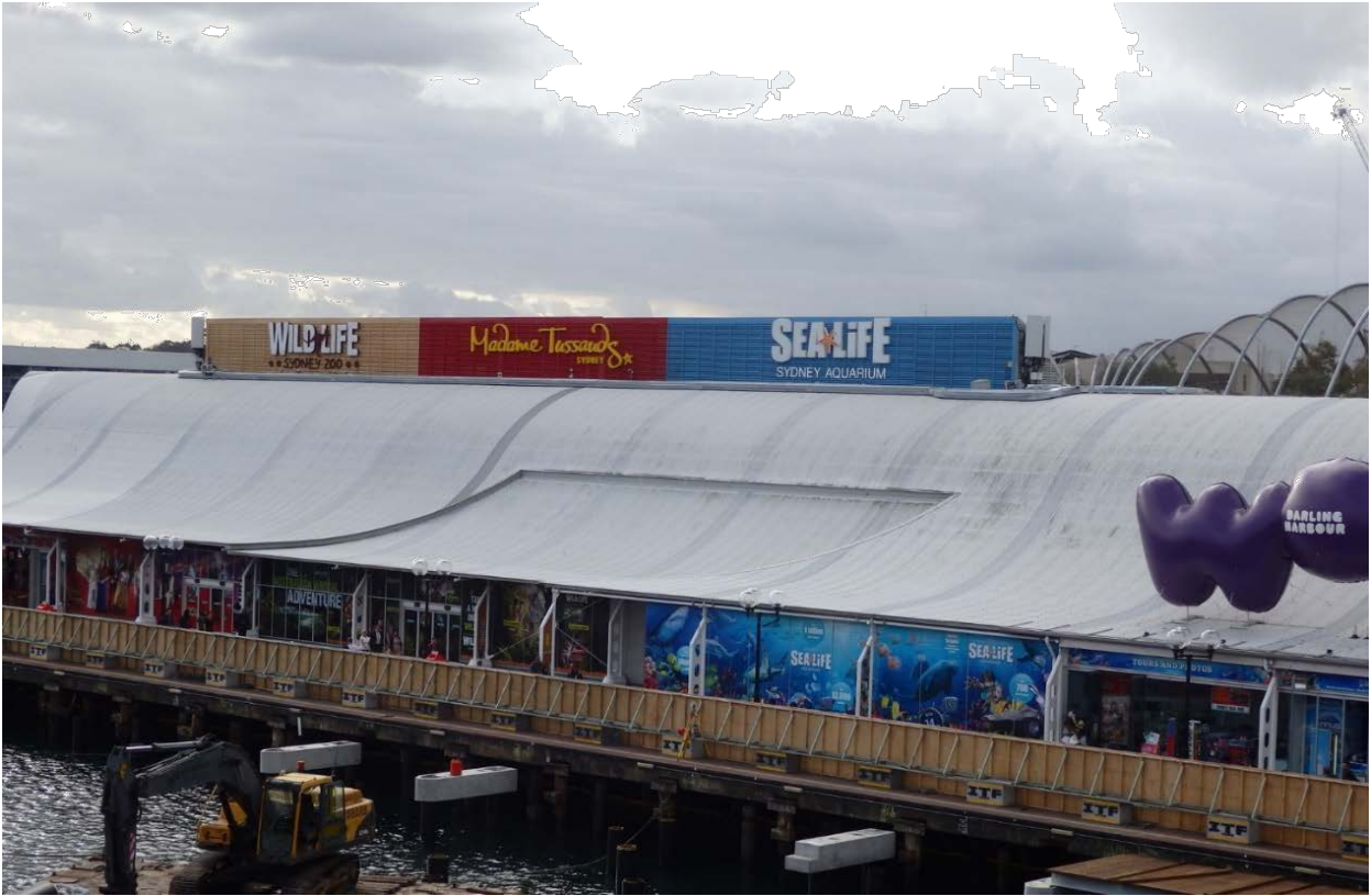
Figure 4 - A rooftop installation that does not break the ridge or overall height of the building
