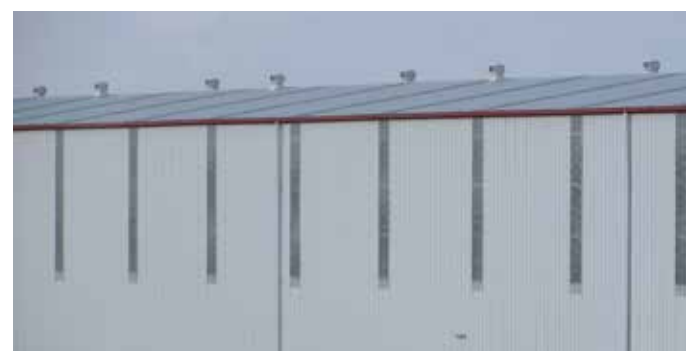
Figure 45 - Translucent sheeting can provide variation to a facade and can facilitate passive heating and lighting
