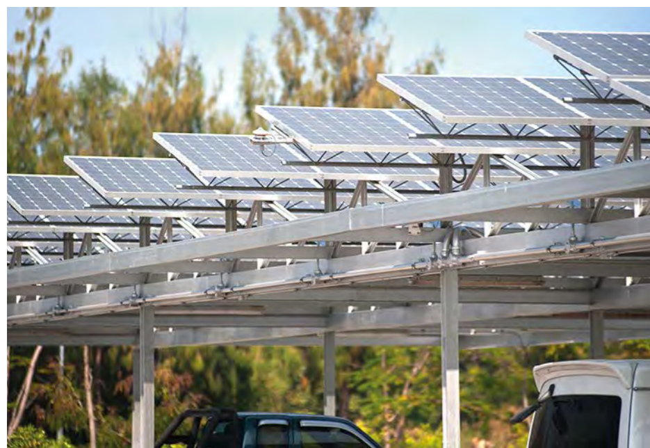
Example of solar carport which will get free energy from the sun, but also incorporate shade protection for the carpark as a bonus
