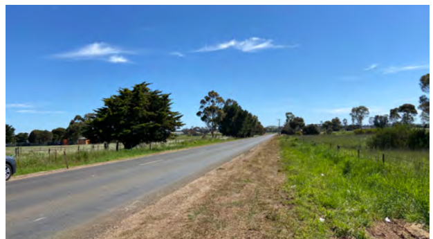
Leakes Road view north
