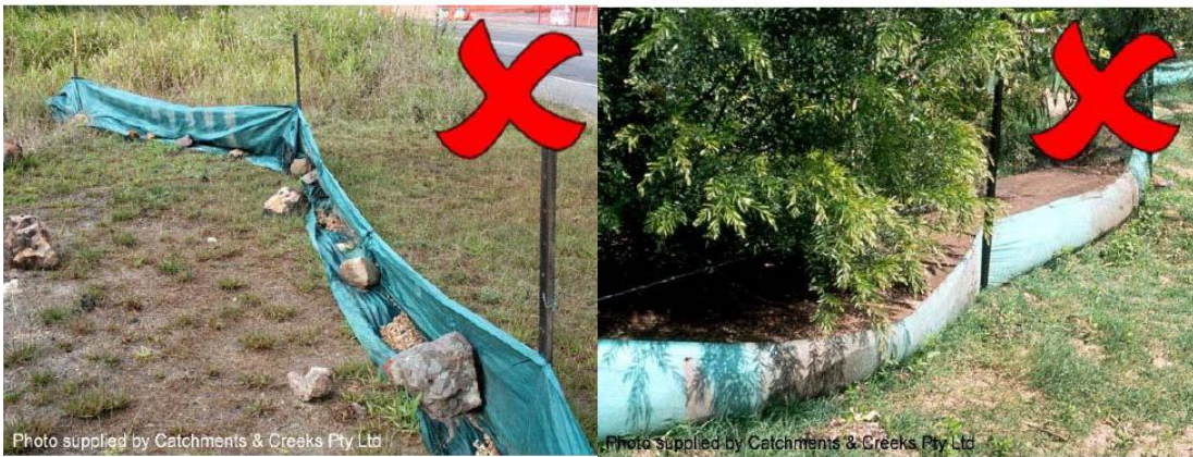
Plate 2: Photo of sediment fences installed correctly (e.g. Sediment fence not securely installed and the sediment fence hasn't been cleared after a storm)
