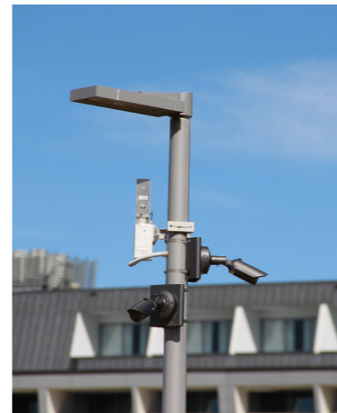
CCTV & Light Post
