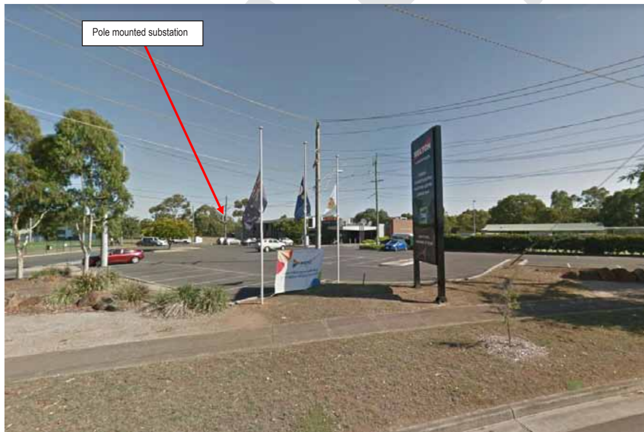
Fig 7 Existing pole mounted substation supplying the Country Club
