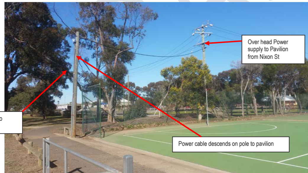
Fig 4 Existing incoming power supply from Nixon Street
