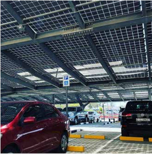
Image 29 Example of solar panels covering car parks which will reduce ambient temperatures
