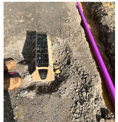
Recycled water pipework in oval
