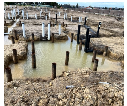
Nov '22– waterlogged pavilion
