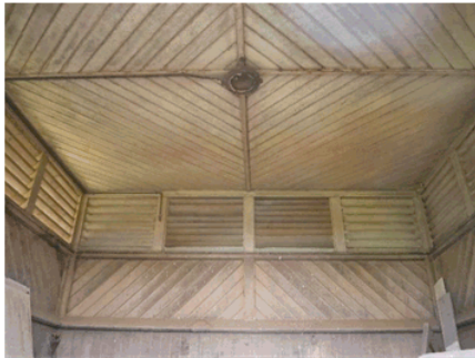
Figure 11 Stallion Box - Interior
