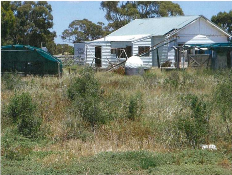
Figure 4: Dilapidated weatherboard house, view towards south
