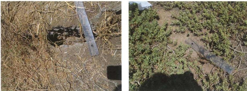
Figure 2: Examples of shrinkage cracks, some of which have apertures greater than 100 mm
