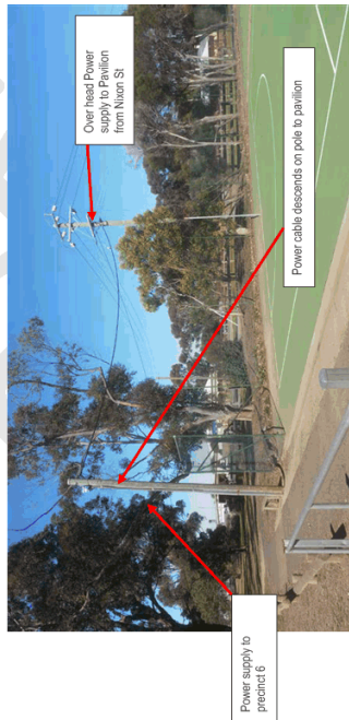
Fig 4 Existing incoming power supply from Nixon Street
