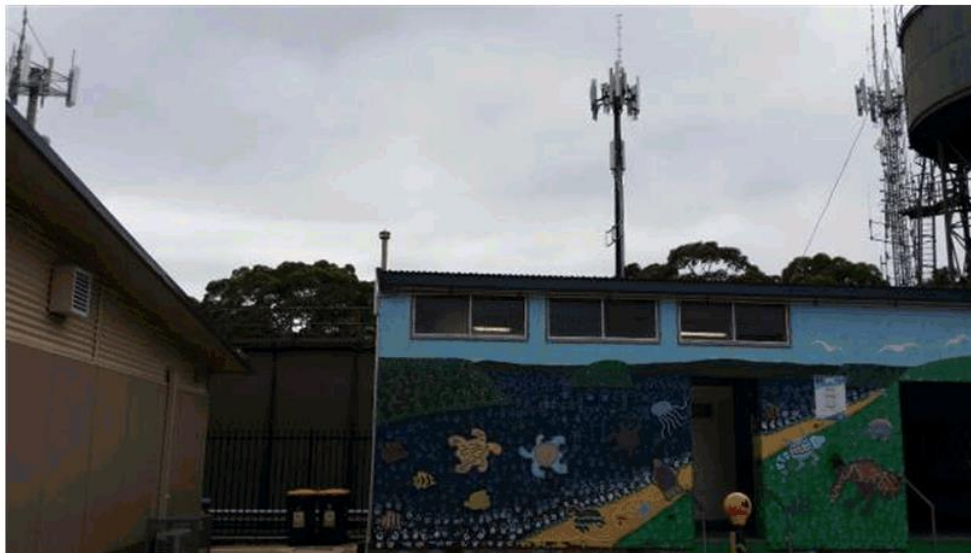
Figure 5 - Two monopoles and a lattice tower, all on the same site, within metres of one another.
