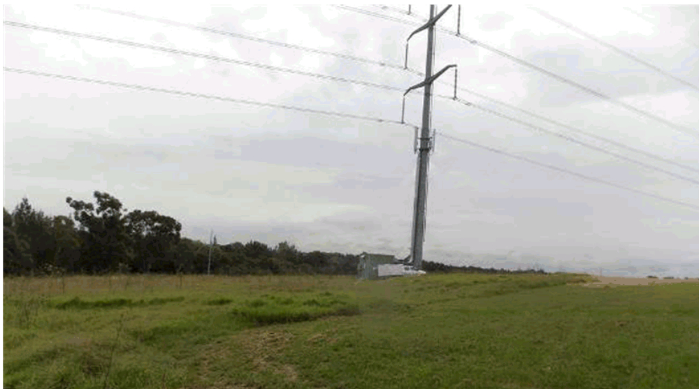
Figure 1 - A co-location installation on a high-voltage electricity pylon.
